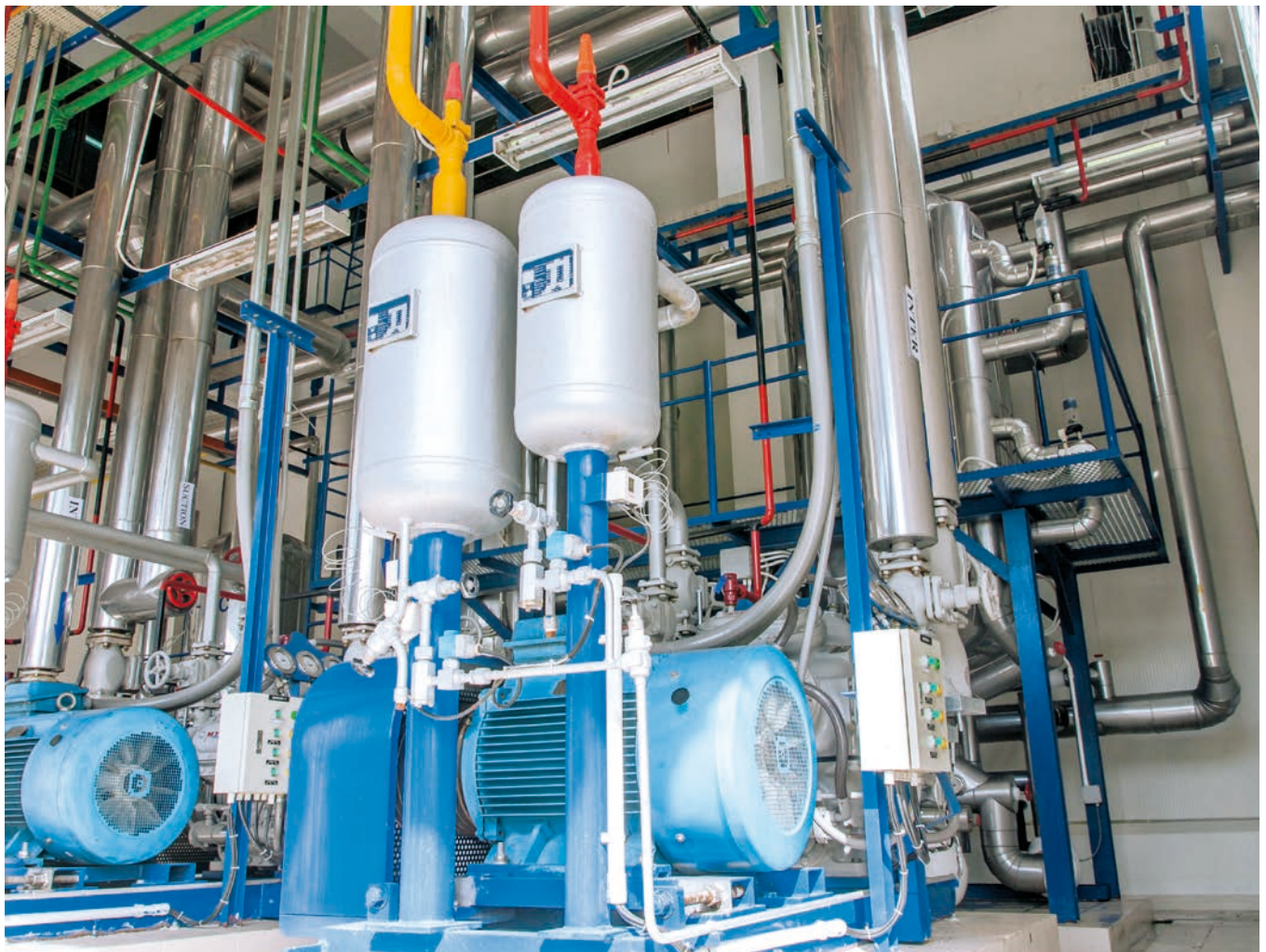
Condition monitoring of compressors
